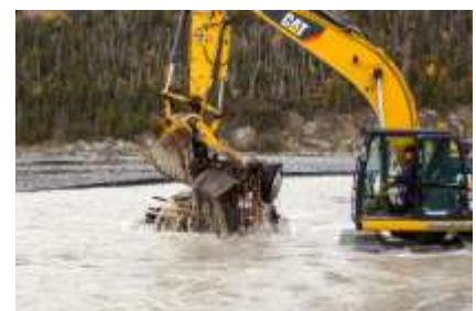
An RV Chassis is extracted from the Kotsina River at our fall cleanup with Copper River Watershed Project and Cruz Construction.
